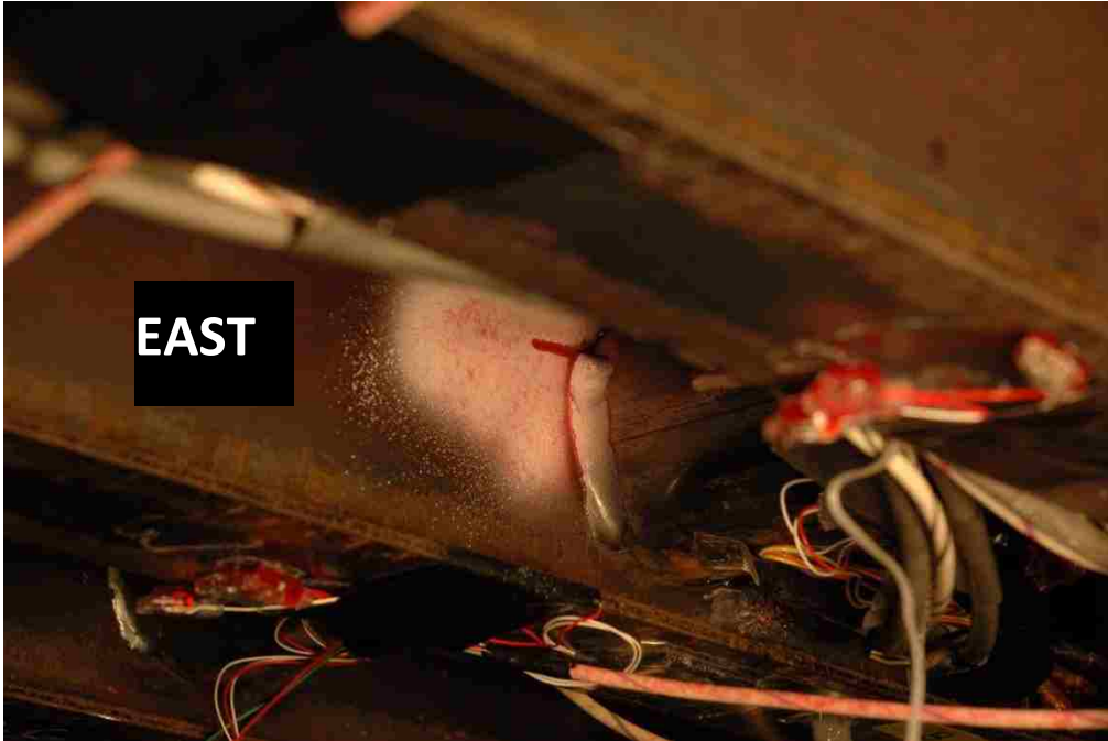
Figure 60. Specimen #1, crack at the east weld of the S5-T2 intersection
