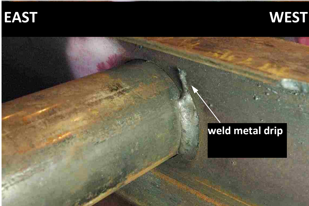
Figure 74. West weld at intersection of S8-T2 in specimen #1
